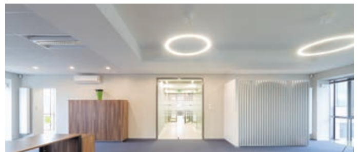
Applied luminaries: Tondo Led, Agat Pos with perforated mesh and louver
