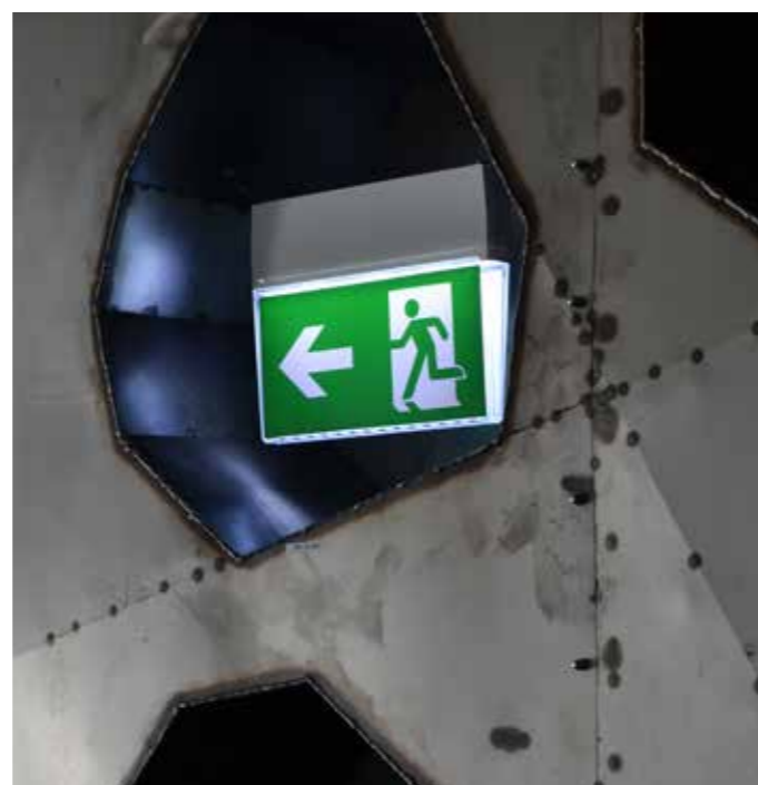
Realisation: Evacuation luminaires of LUXIONA
